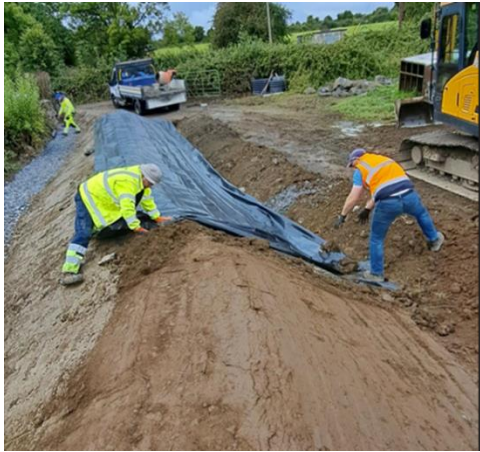
OPW FUNDED FLOOD PROTECTION MEASURES TO HOUSE AT ROO BEING INSTALLED BY THE LOCAL ROAD STAFF IN GORT
