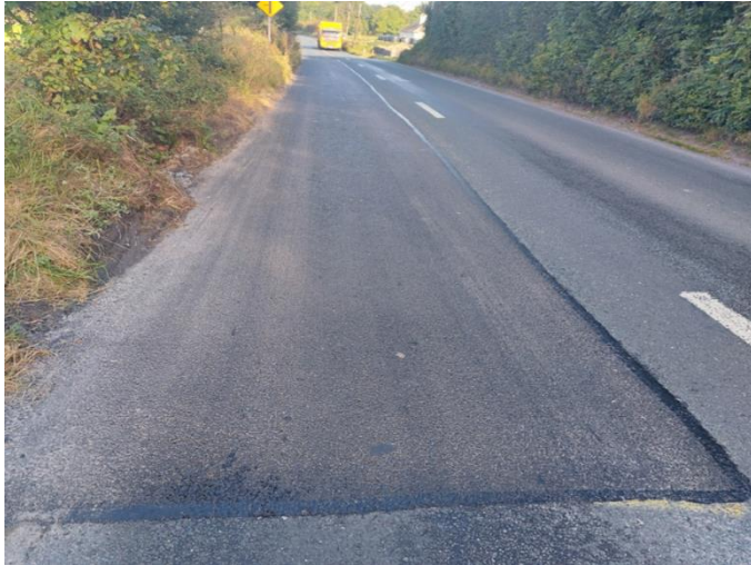
COLLAPSED ROAD PATCHES
