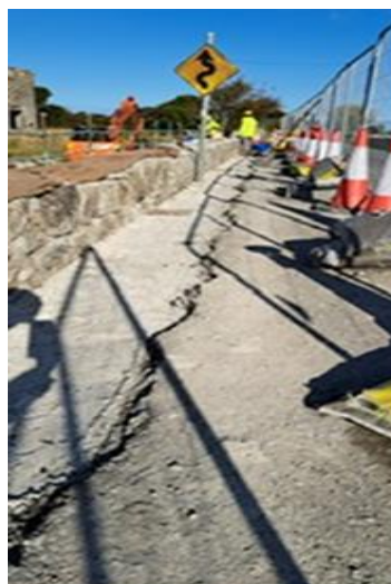
SEVERE WEATHER EMERGENCY WORKS -TAWNAGH WEST CAUSEWAY/BRIDGE REPAIR ON ACCESS ROAD TO TRAUGHT BEACH
