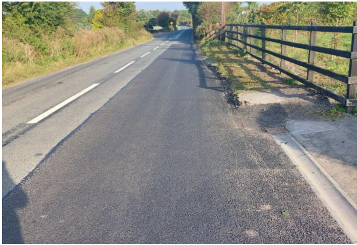
COLLAPSED ROAD PATCHES
