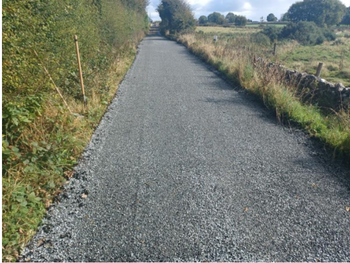
OPW MINOR DRAINAGE WORKS SCHEME BEING COMPLETED AT CARROWNAMORRISSEY, KILCONIERIN TO RELIEVE LONG-STANDING ISSUE ON THE ADJACENT REGIONAL ROAD. WORKS BEING UNDERTAKEN BY THE LOCAL ROAD STAFF IN LOUGHREA
