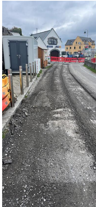
DEPARTMENT OF RURAL AND COMMUNITY DEVELOPMENT FUNDING WORKS BEING UNDERTAKEN ON CILL RÓNÁIN INIS MÓR
