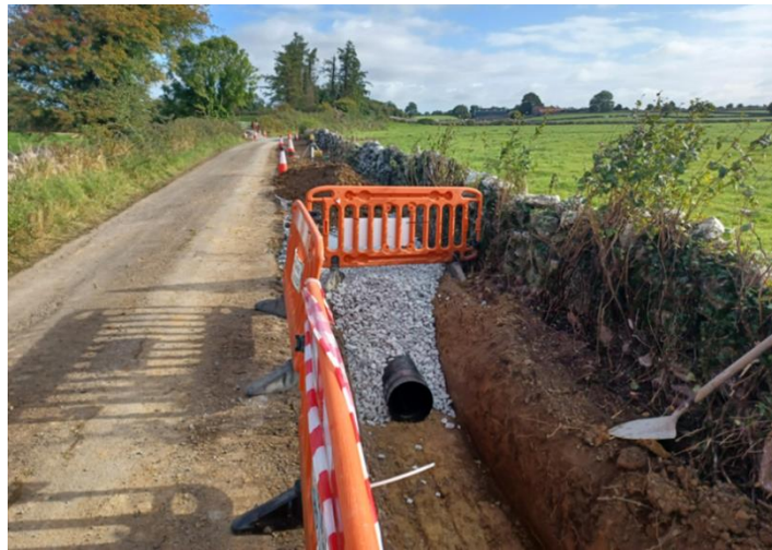
ONE OF EIGHT ROADS REPAIRED UNDER THE LOCAL IMPROVEMENT SCHEME WITHIN THE LOUGHREA MD
